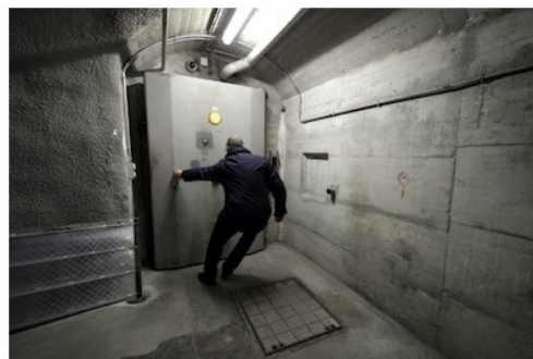
Deltalis' Patrick Mueller opens a bunker door of the Deltalis Swiss Mountain Data Center , a former Swiss Army bunker built in the Alps during the Cold War, on November 18, 2013 near Attinghausen, Central Switzerland. With the world still shaking from repeated data leak scandals and fears of spies lurking behind every byte, Switzerland,
