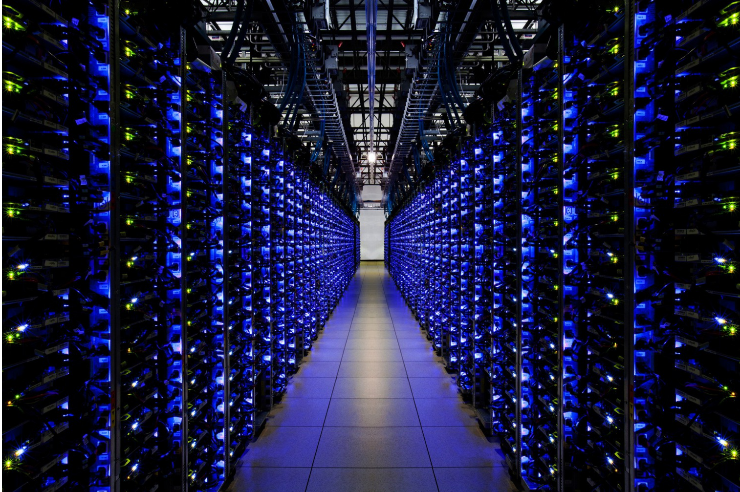
Google data center
